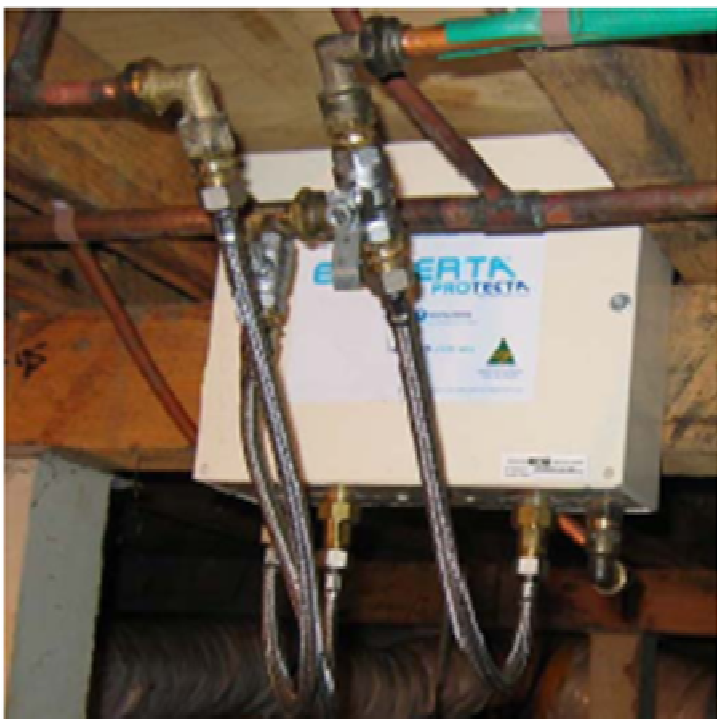
Ecoverta Protecta Under-Floor-Installation, note by-pass line hard plumbed for external garden use.
