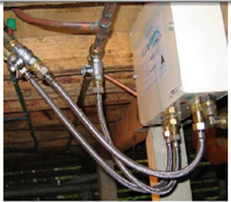
Ecoverta Protecta Under-Floor-Installation, note shut-off valves on both hot and cold supplies to unit.
