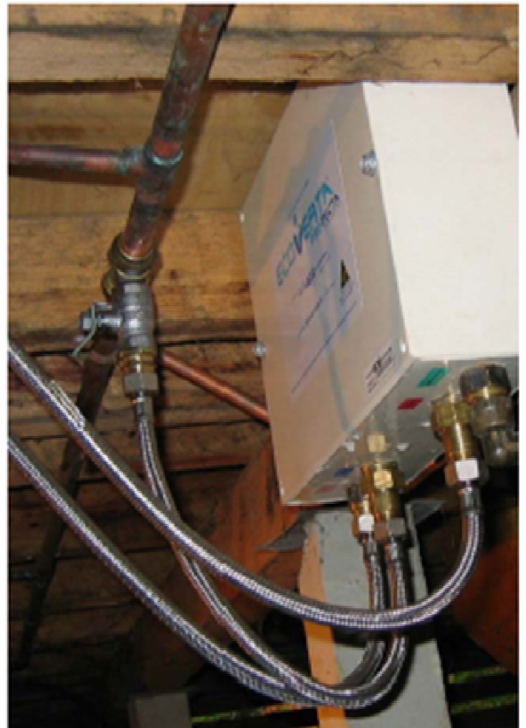
Ecoverta Protecta Under-Floor-Installation, note Braided supply lines for ease of install.
