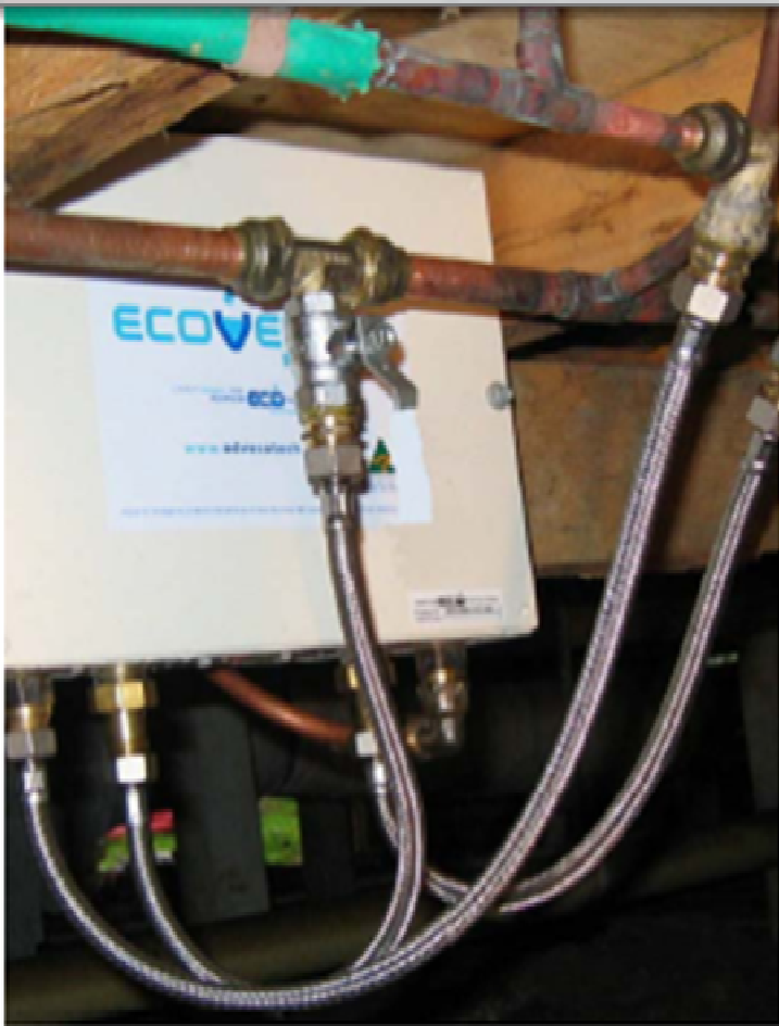
Ecoverta Protecta Under-Floor-Installation, note temperature control cold supply branched off original
