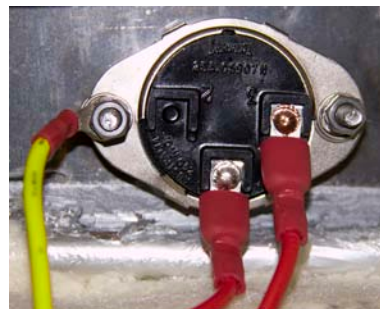
Thermostat Connection Push on connectors Earth to Earth lug Ensure earth connection is tight.
