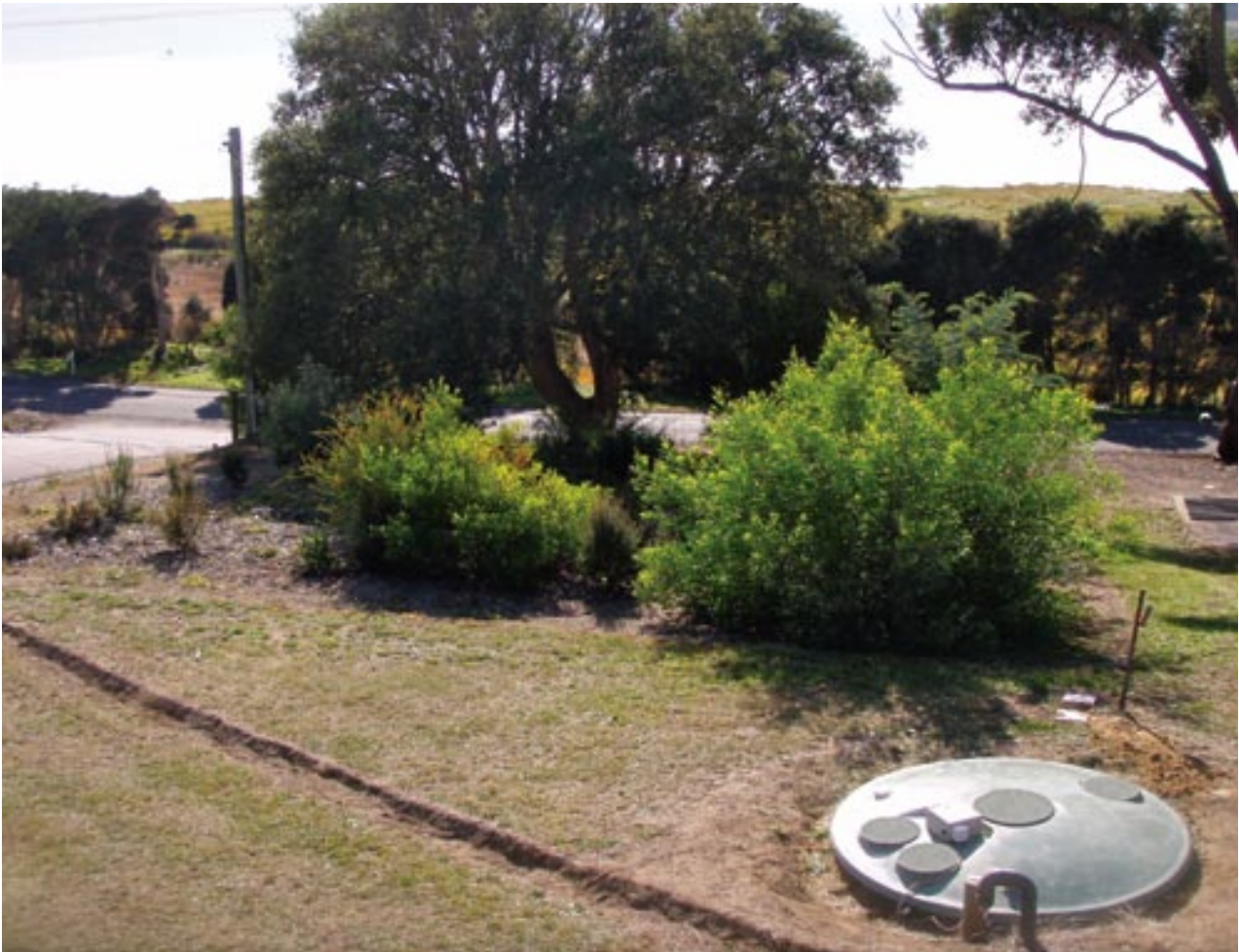
Typical installation - note cutoff drain protecting irrigation field.
